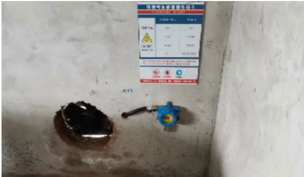
Alarm for Combustible Gases in Hazardous Chemicals Warehouse
