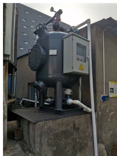
Filtration and Purification Equipment – Shallow Medium Filter
